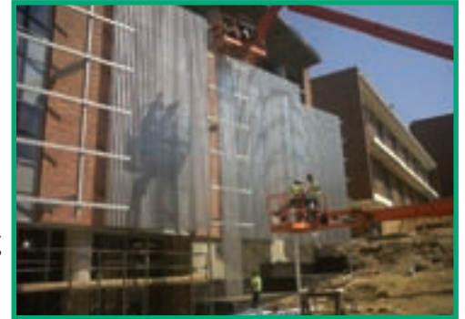
Stainless steel panels being installed at the Georgia Tech Undergraduate Learning Center
